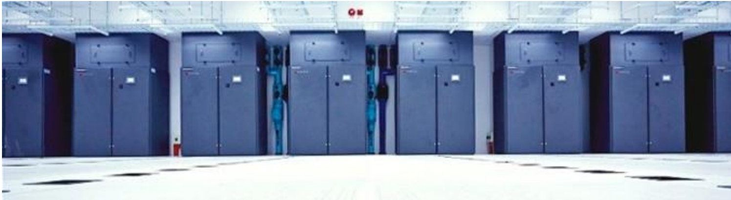
Cloud service providers' data centre requirements continue to grow
