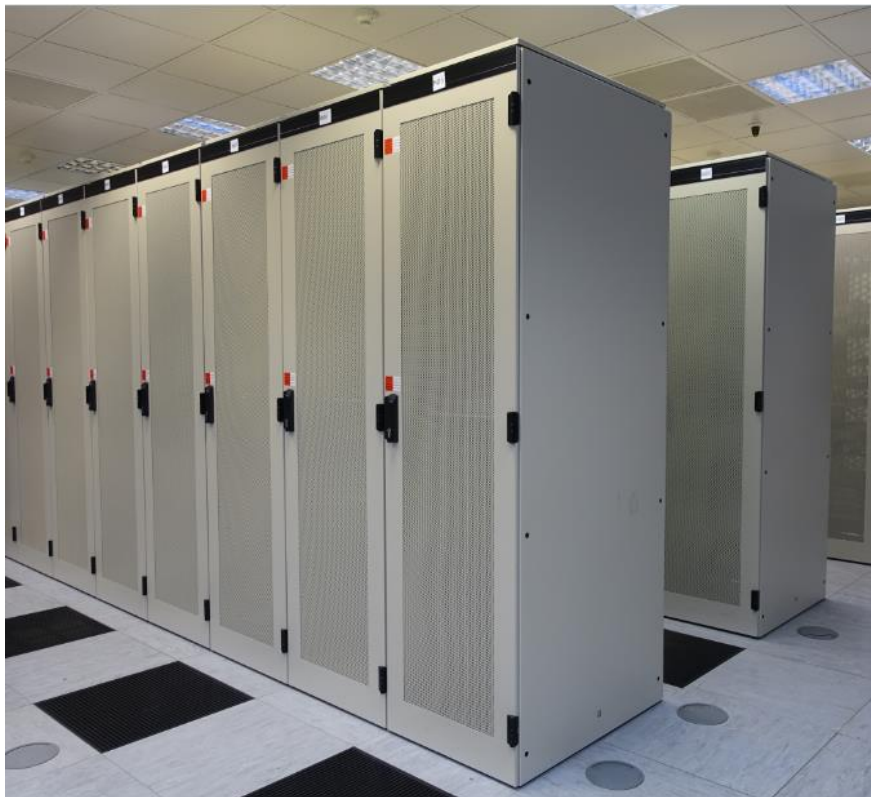
Data centre interior
